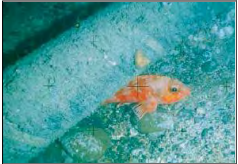
126mm diameter power cable in Submarine Cable Protection Zone across Cook Strait, NZ
